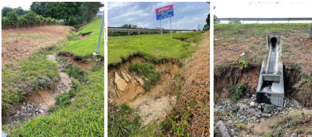
Severe Ditch Erosion
